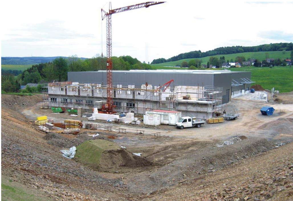
Construction status of the sales and service center in Meinerzhagen on May 11 th , 2009.
